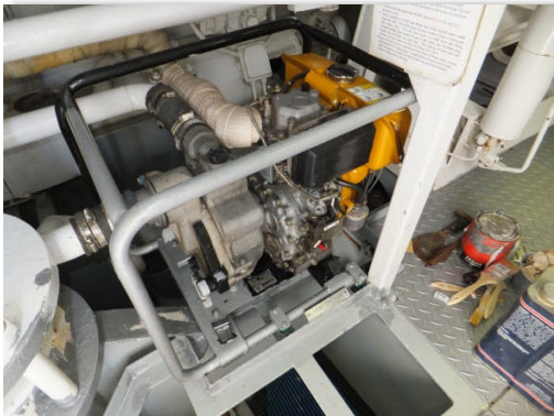
Diesel Fire Pump
